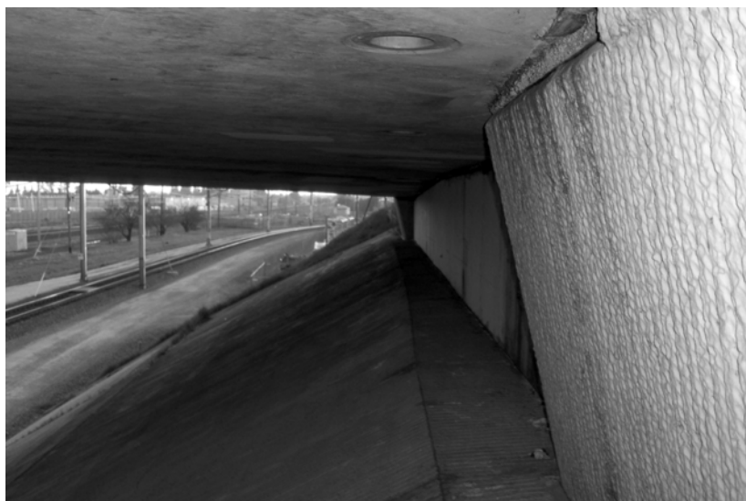
Figure 1. Sloped abutment at west side of the Arden Way overpass of railroad tracks in Sacramento, California. Note weep-hole entrances to bridge nesting chambers in upper foreground. Weep holes here are 0.8 m (2.3 ft) away from the 1.6 m (5 ft) tall vertical abutment wall. One of these holes adjacent to the abutment wall was used in three different years by Northern Rough-winged Swallows.
